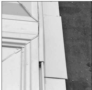
FIGURE 2B – ONE SIDE OF A STACKED UNIT COMPLETED. SILL WOULD BE SIMILAR
